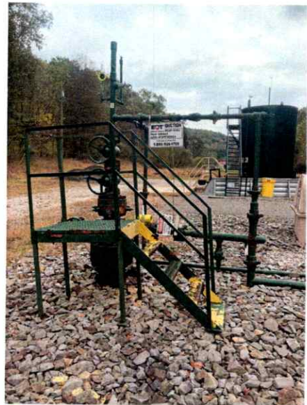
OXF 47 Well Looking Southeast
